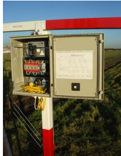
Control Box on Base Post
